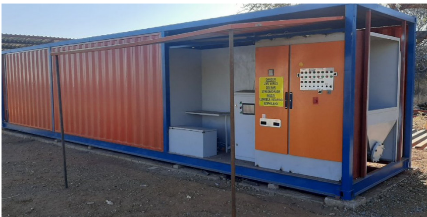
Figure 8. Electrical and control system panel
