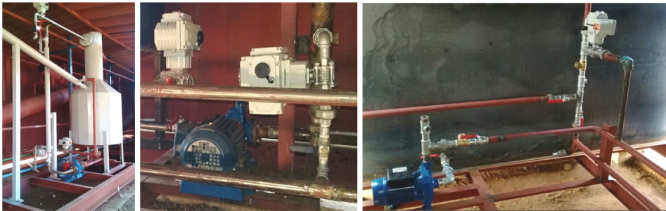
Figure 7. Knock-out drum, heat-exchangers, valves, pumps, and piping.
